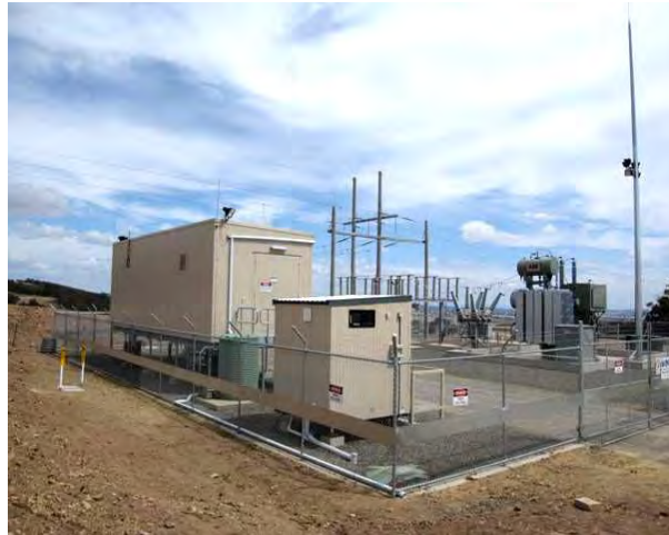
Plate 8 – Typical wind farm collector substation (Source Epuron 2009)
