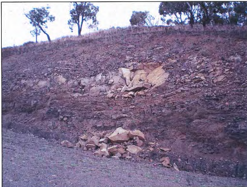
Rock Failure Along Abercrombie Road, Adjacent To Southern Central Site Boundary
